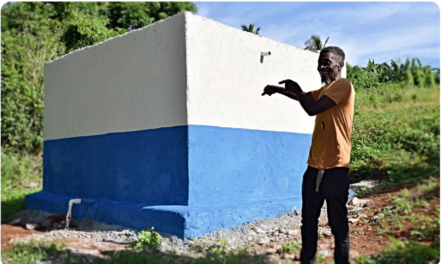
With UN support a community holding tank was constructed in rural Mount Airy, benefiting diverse groups of women farmers
